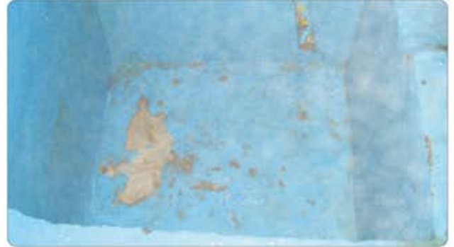
Cracked surface for Concrete water tank after 3 years installation
