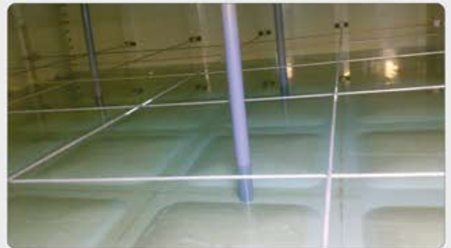
Inside state of Esinoks GRP Water tank after 3 years installation
