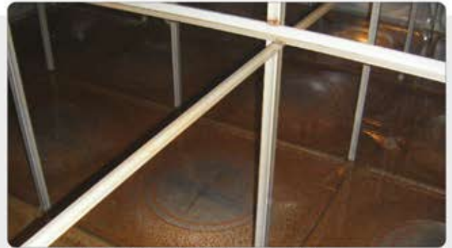
Rusted steel for STS Water tank after 3 years installation
